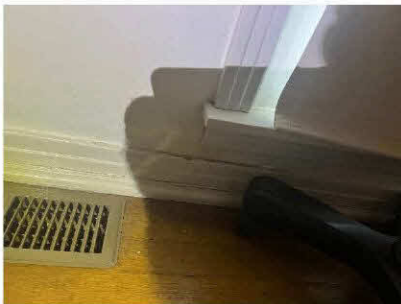
water damage on windows
