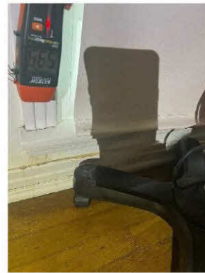
Water damage on window
