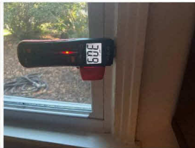
Moisture of window
