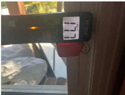
Moisture of window
